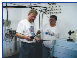
South Alabama D-STAR Repeater Installation
